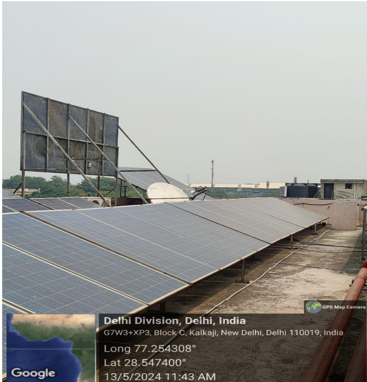
Solar panel installed on rooftop at JIMS kalkaji
