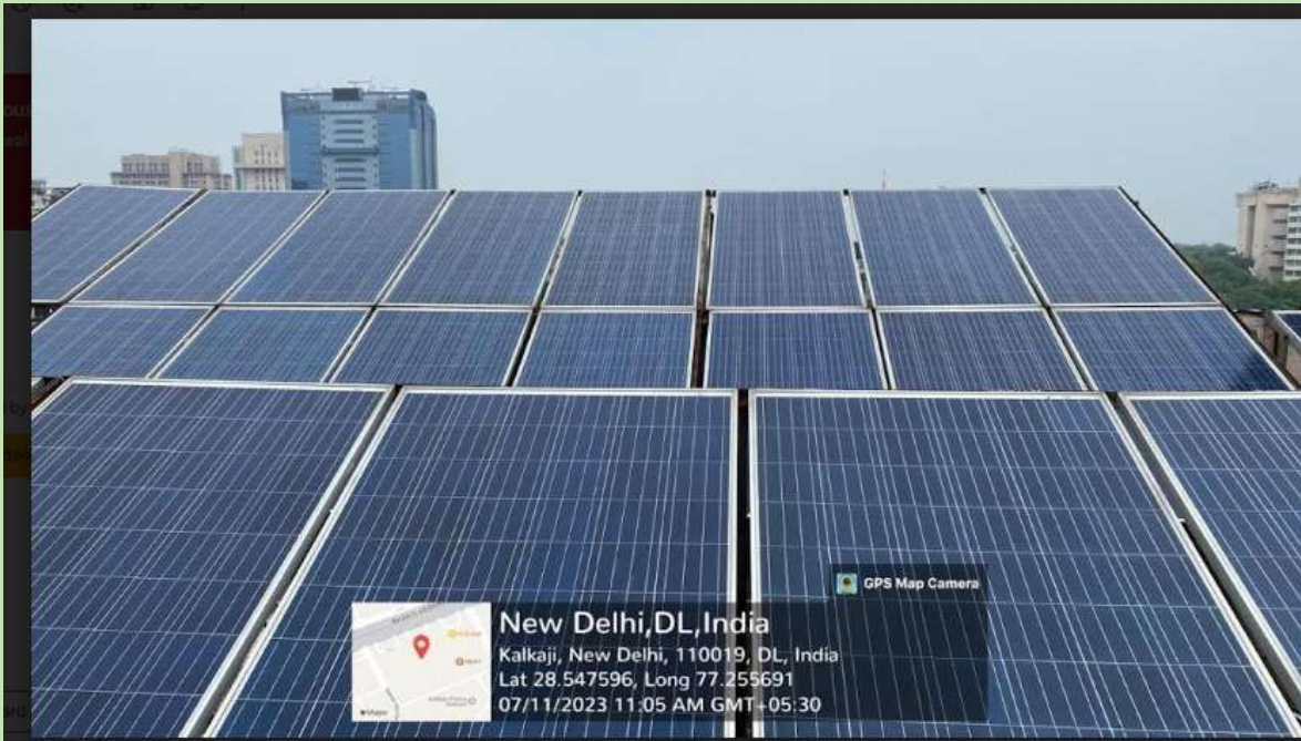
Solar Panel Installed at JIMS Kalkaji
