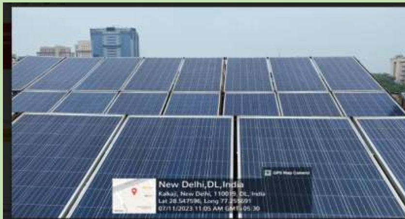
Solar panel installed at JIMS Kalkaji
