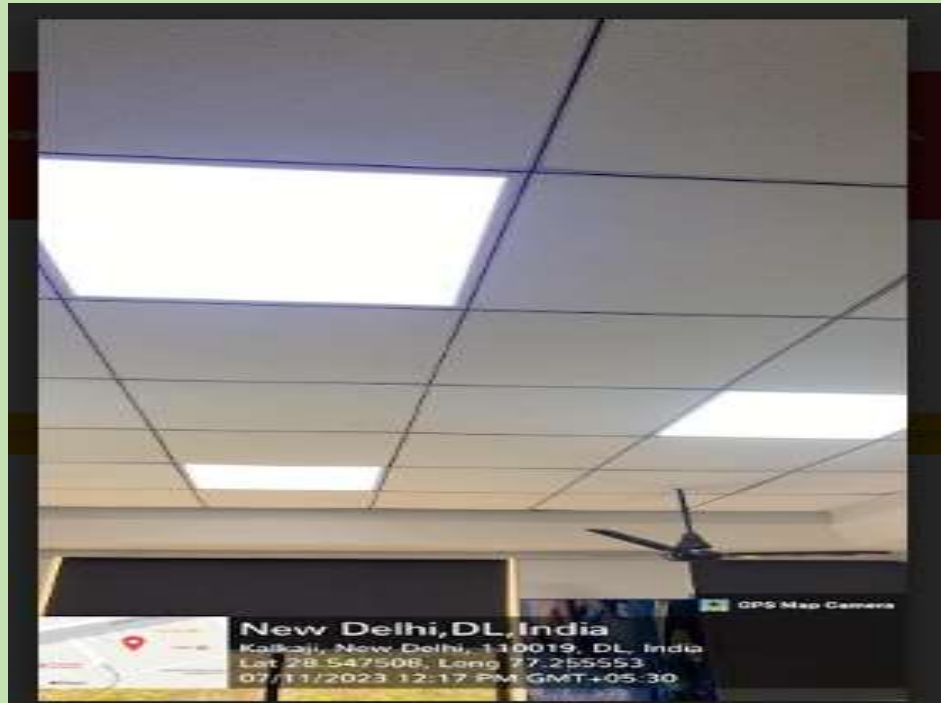
LED Lights installed at JIMS Kalkaji (Classrooms & Corridors)
